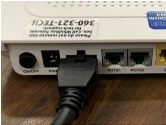
UPS power cable connected to the ONT
